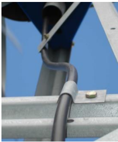
PHOTO 7 – HOSE BRACKET [HBK] INSTALLED ON M23 WITH AIRLINE INSTALLED (VIEW FROM BOTTOM OF TOWER)
